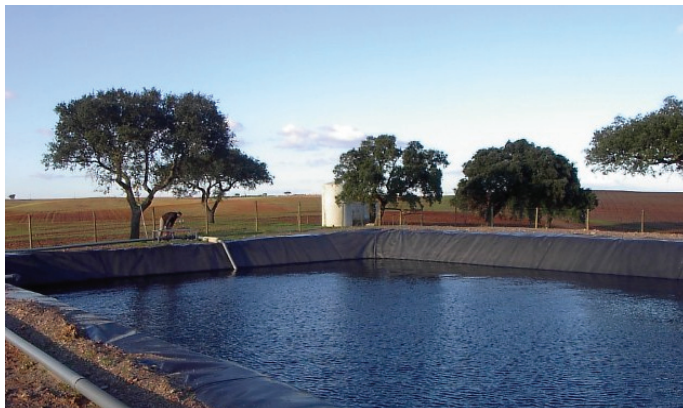
Fig. 14. Wastewater treatment system at Mingorra
