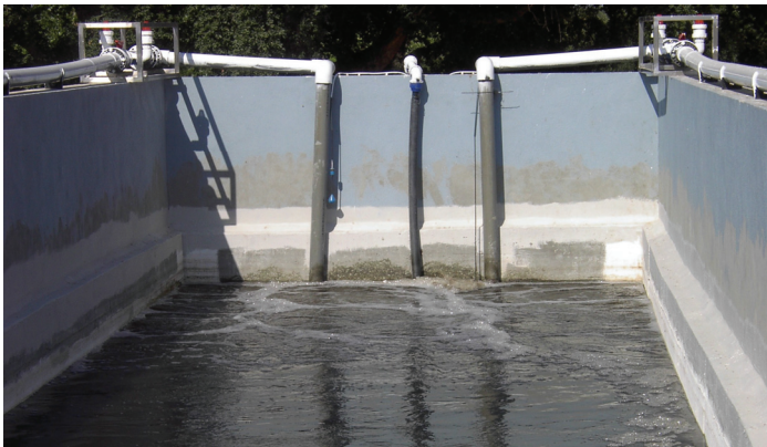
Fig. 13. Wastewater treatment system at Catapereiro
